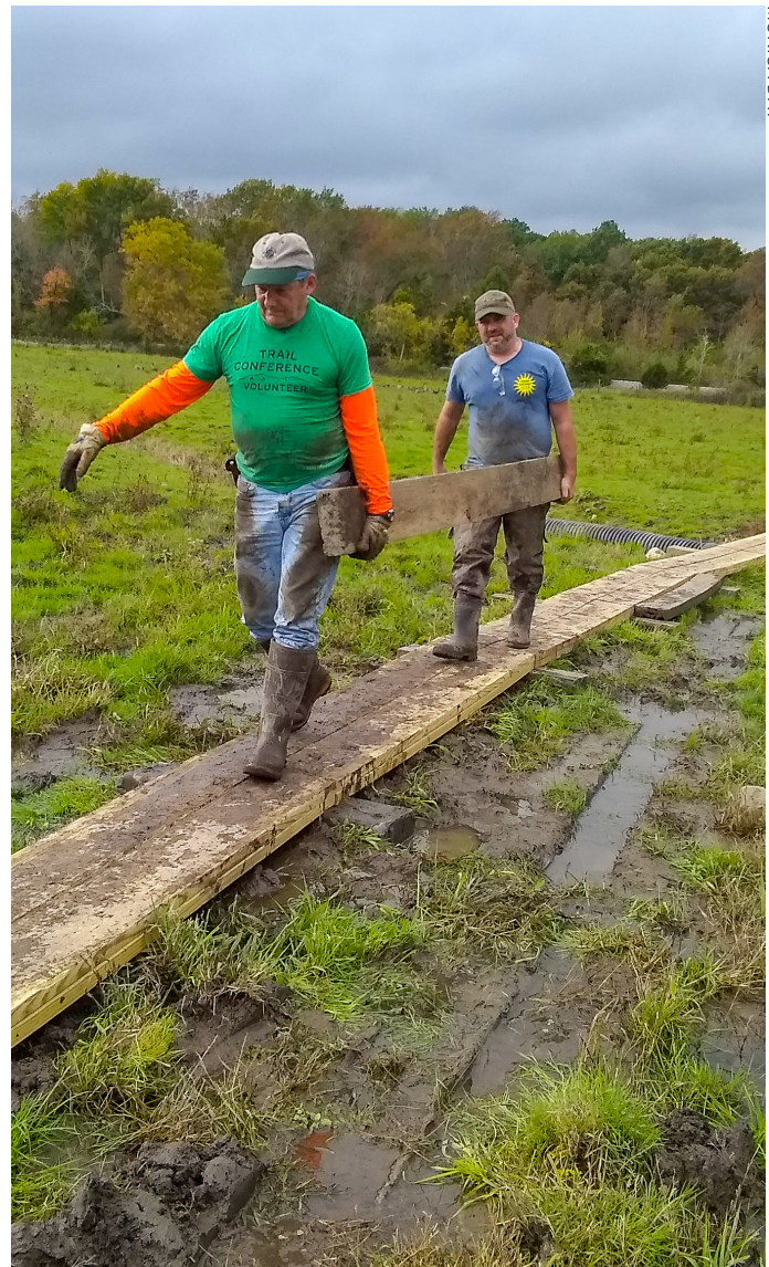
The West Jersey Crew worked six weekends replacing planking on the Pochuck section of the A.T.
